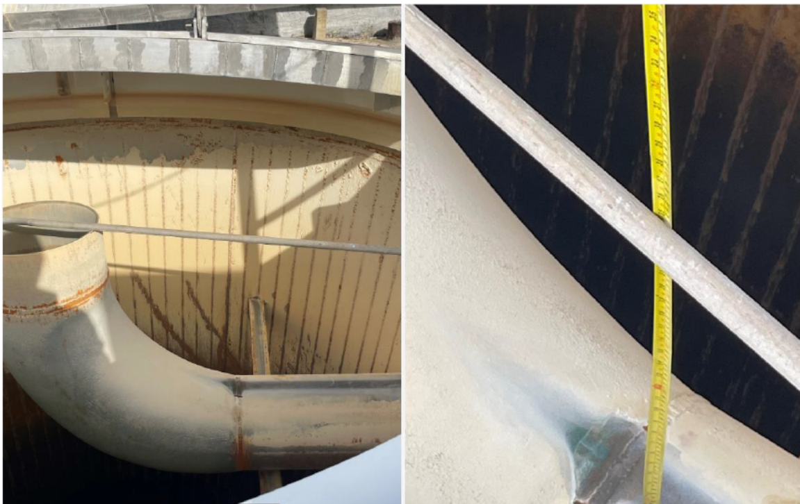
Exhibit 2-3b. Spiractor Effluent Pipe in Place
